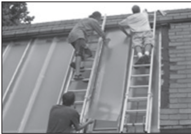
Evan Coughneour, Nathan and Simon Dorsett help install KaiWall on UFM Solar Addition, 2007.
